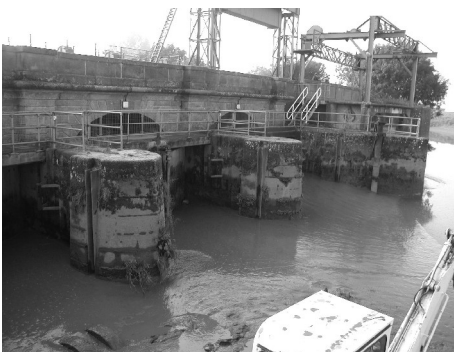
Above: 4 metres of silt against the gates in 2006
